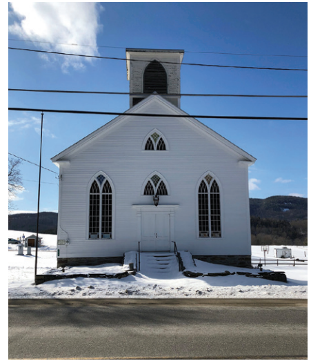
Starksboro Starksboro Village Meeting House Society 5,000 Starksboro Village Meeting House window restoration
