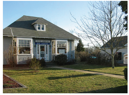
West Harwich Chase Library Association, Inc. • 4,812 Chase Library exterior painting and repairs
