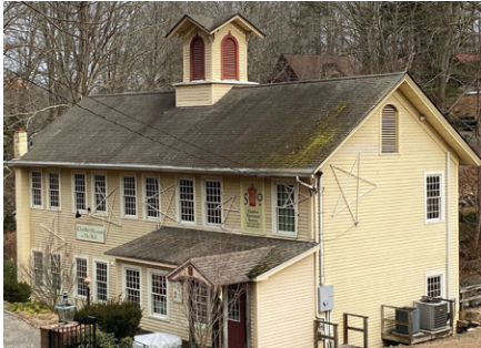
Chester Chester Historical Society • 5,000 C. L. Griswold Mill cupola and roof repairs
