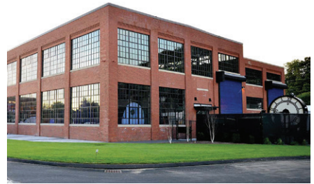
Providence WaterFire Providence • 9,500 WaterFire Arts Center (former U.S. Rubber Company warehouse) masonry repair
