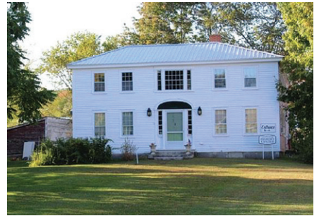
Tamworth Tamworth History Center • 3,450 Hall-Dyer House exterior painting, clapboard repair, window restoration
