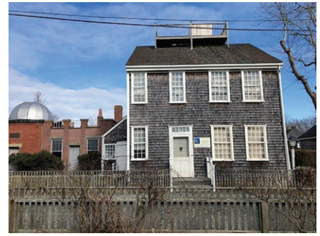
Nantucket Maria Mitchell Association • 8,250 Maria Mitchell House exterior painting, window sash reglazing
