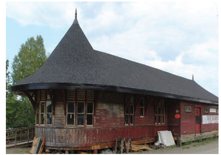
Greenville Friends of the Greenville Junction Depot • 6,000 Canadian Pacific Railroad Depot exterior rehabilitation
