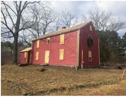
Canton Canton Historical Society • 3,480 David and Abigail Tilden House fire detection/ security system installation
