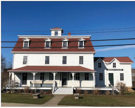
Block Island Block Island Historical Society • 9,500 Woonsocket House cupola repair and restoration
