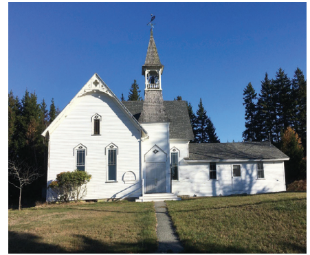
Swan's Island Swan's Island Historical Society • 6,000 Swan's Island Methodist Church foundation repair
