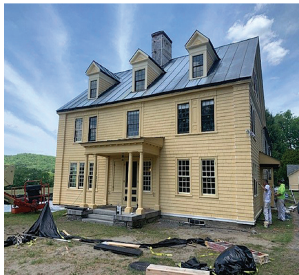
Cornish Opera North • 7,500 Charles Beaman House roof painting, storm sash restoration, porch repair
