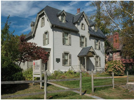
Hartford Harriet Beecher Stowe Center • 9,000 Harriet Beecher Stowe House bay window restoration
