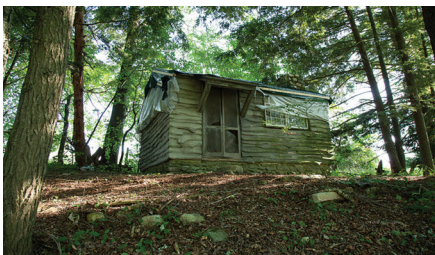
Great Barrington James Weldon Johnson Foundation • 10,000 James Weldon Johnson writing cabin chimney, foundation, and roof repair
